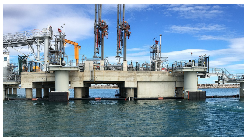
Installed permanent boom system
